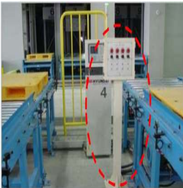
▶ Conveyor Operation Panel
