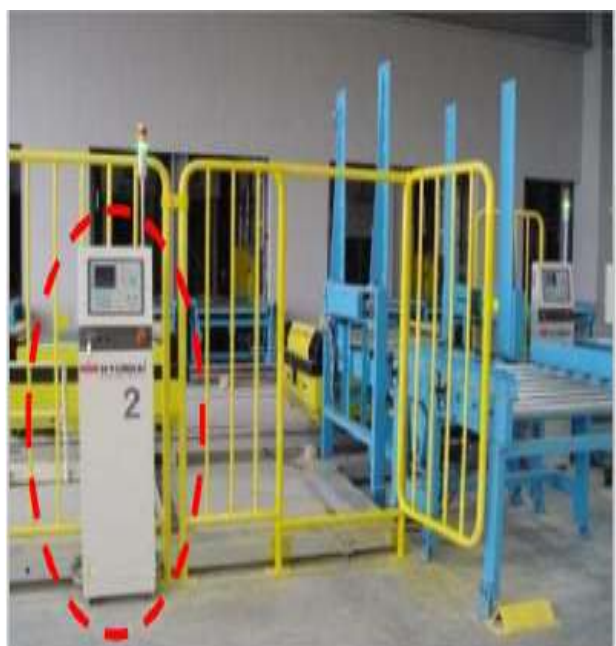
▶ Stacker Crane Operation Panel
